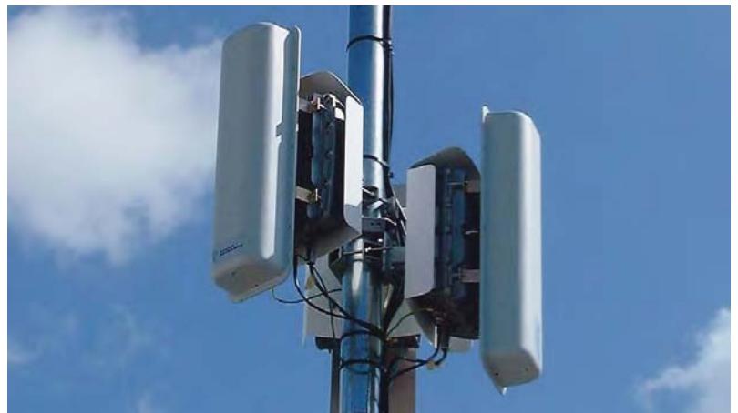
HiperMAX mast head units deployed in Vodafone Malta
